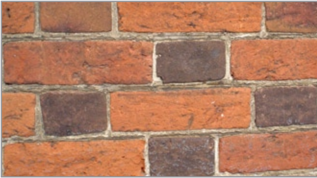
This wall in Potton is built of typical Oxford Clay bricks with their variation in colour, due in this instance to different oxygen levels in the kiln during firing.
