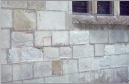
The Totternhoe Stone is 'spalling' (peeling away in layers). Each winter water that has seeped into the porous rock freezes and expands, forcing off a layer of rock. The acidity of the rain also decomposes the limestone, causing it to crumble.
