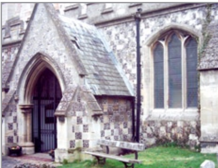
Houghton Regis Church. This elegant chequerboard pattern is made up of alternating Chalk Rock and flint.
