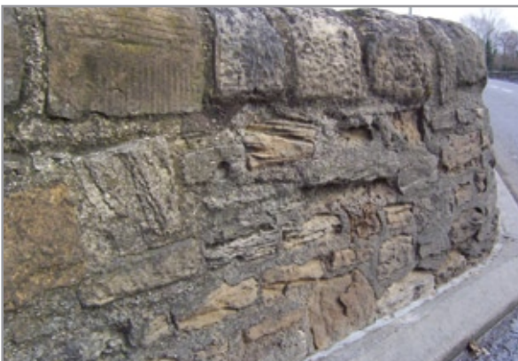
Bromham Bridge is a Scheduled Ancient Monument dating from the 13th century with extensive 15th and 19th century repairs. It is built of the local oolitic limestone with some 19th century Portland Limestone and brick.
