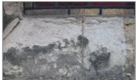
Below, a Totternhoe Stone windowsill weathered by rain and frost action.
